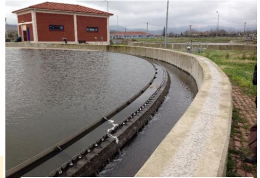
Primary Wastewater Clarifier in Yalova
