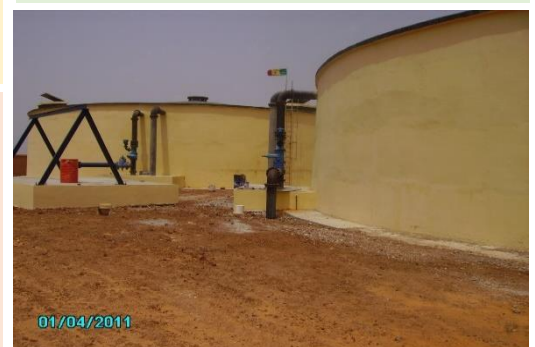
Water reservoir in Tassette
