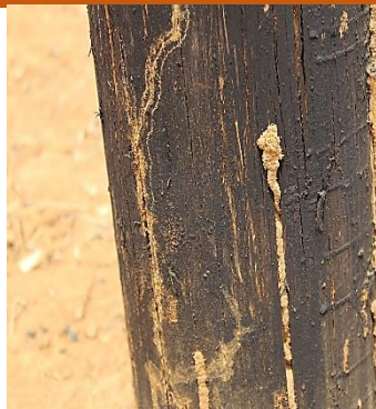
TERMITE INFESTED WOODEN POLES
