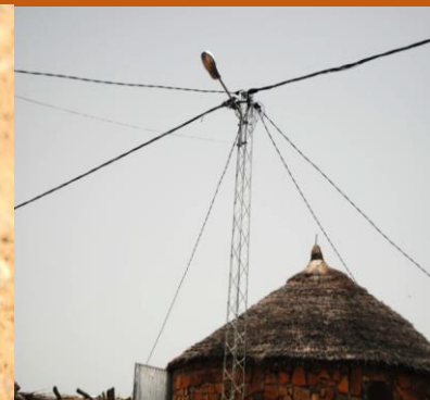
STEEL POLES USED IN NORTHERN REGION
