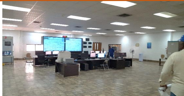
INSTRUMENTATION AND CONTROL SYSTEM AT THE PLANT
