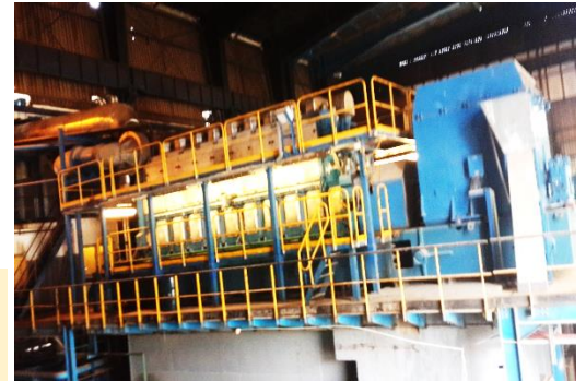
The generator financed by IDB
