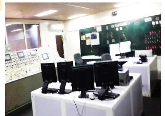
The Control Room of the Power Plant
