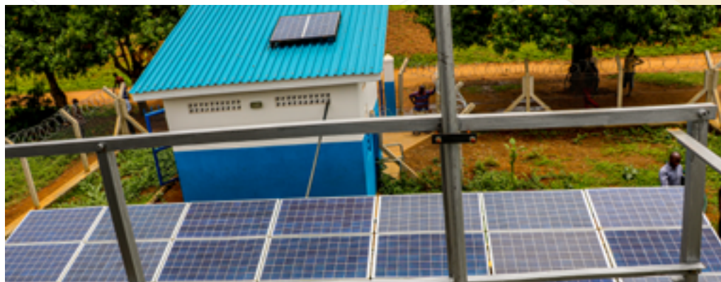
Figure 5: Typical Uganda WSSP mini solar-powered pumping scheme
